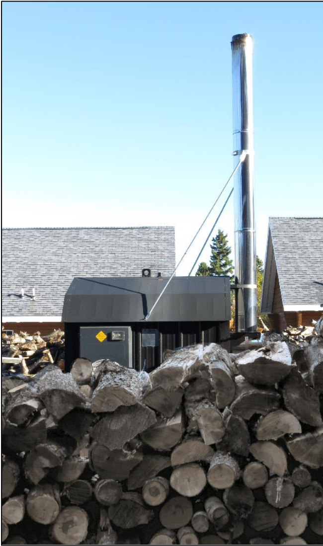
The Mariner North wood-fired district heating micro-grid is powered by a single conventional outdoor boiler, with propane back-up.
