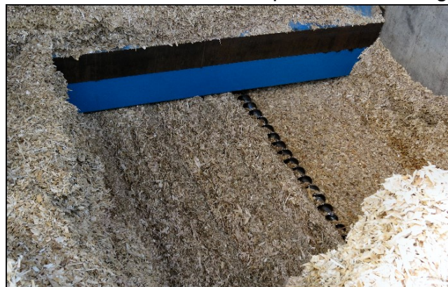
Concrete pit for chip storage and single walking auger.
