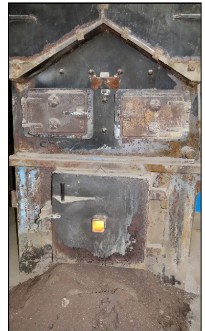
Combustion chamber and boiler.
