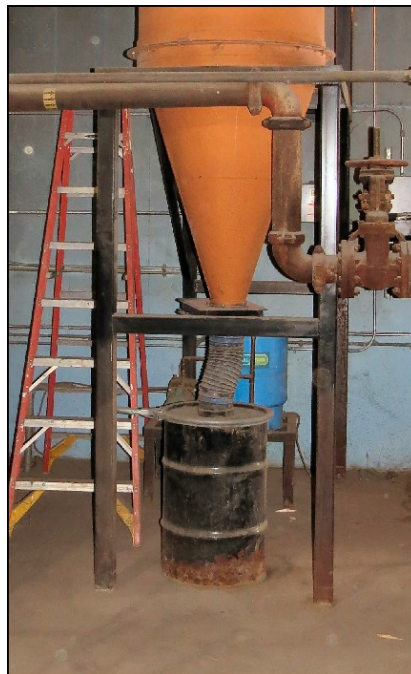
Cyclone separator, to remove particulate matter from the emissions stream.
