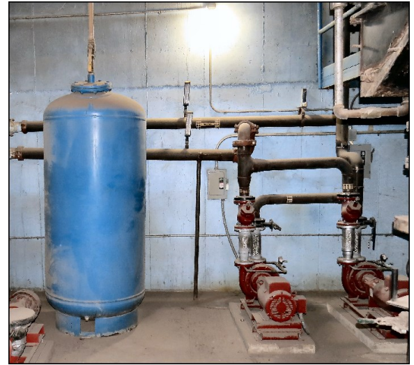
Thermal storage tank and circulation pumps.
