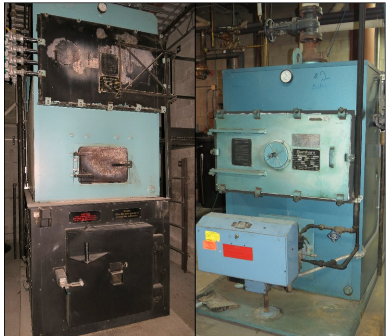
Messersmith boiler unit and control unit.
