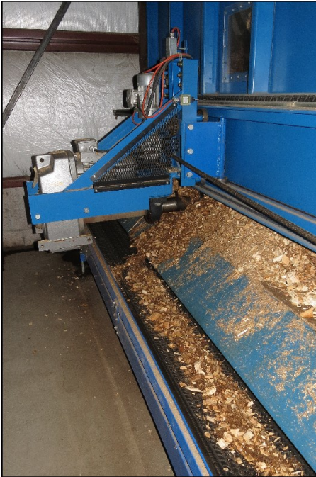
Storage bin/area, traveling auger, and conveyor.
