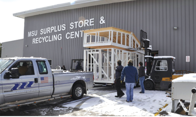
MSU Surplus lifting the loft onto the first floor framing on a snowing spring day in Michigan.
