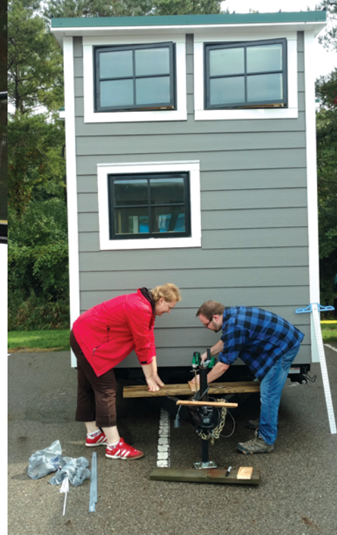
Dr. Rob Dalton and PhD in PDC student Sirle Salmistu installing the tongue deck for the mini-split compressor.
