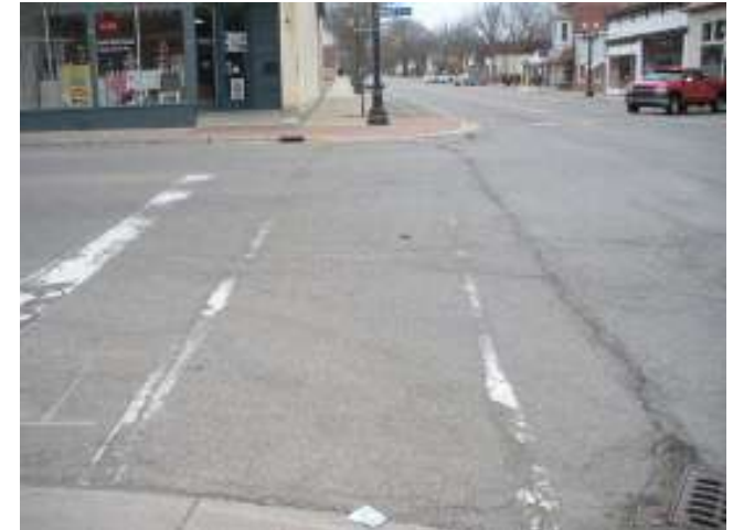
Worn Crosswalk Paint in Downtown, photo taken in March 2009
