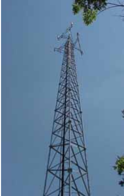
Figure 9: A Base Transceiver Station
