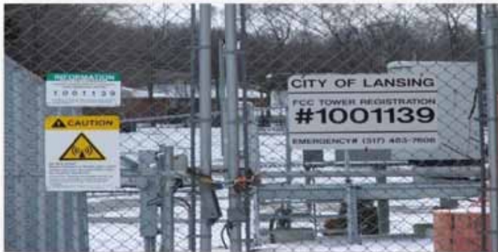
Figure 27: A Caution Sign Posted on the Fence surrounding a Tower Compact Area in Lansing.
