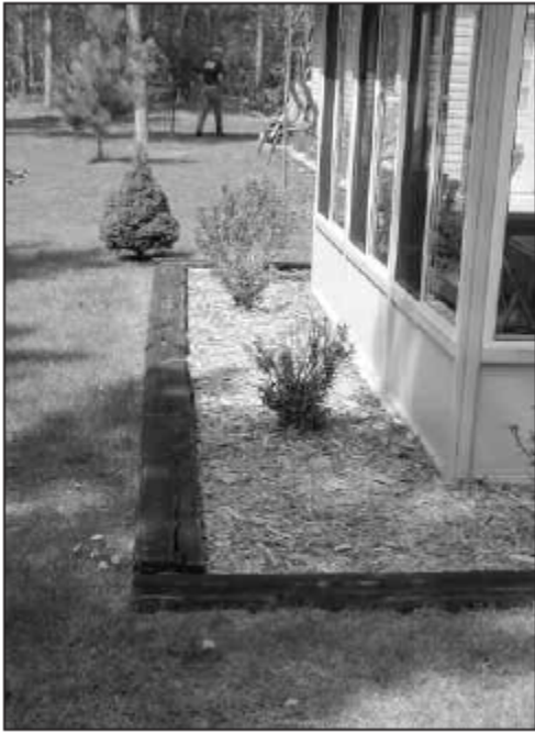
Figure 2 The wood mulch in this photo is flammable and should be replaced with a non-comustible mulch such as limestone, rock or even mineral salt.
