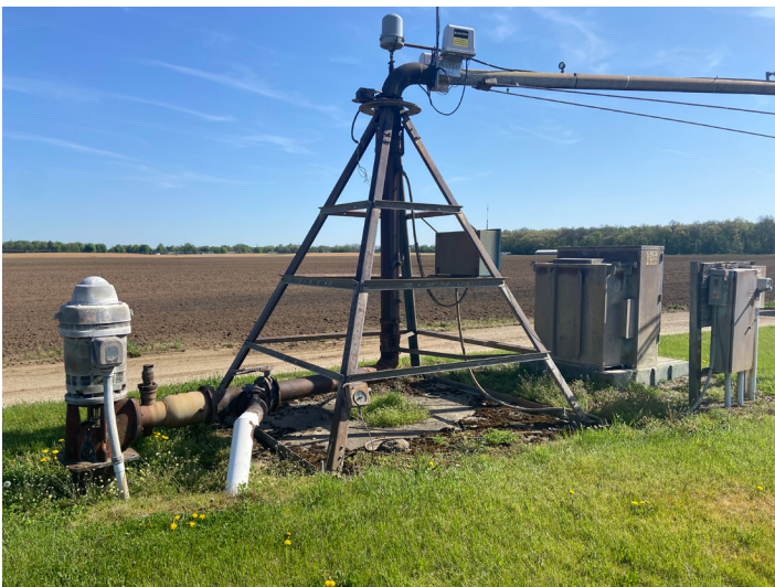
Figure 5. Installed vertical turbine pump system. Michigan State University.
