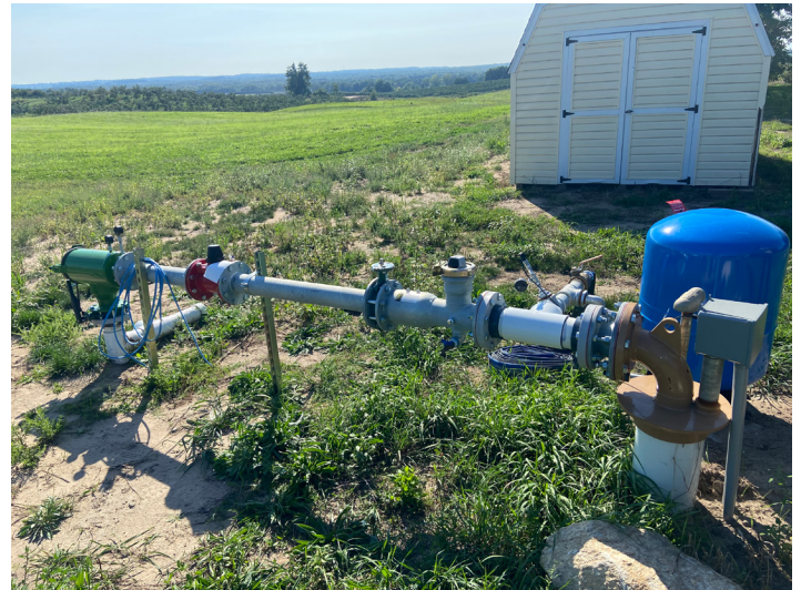
Figure 7. Installed submersible pump system. Michigan State University.
