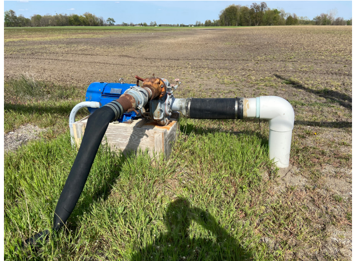
Figure 2. Installed centrifugal pump system. Michigan State University.
