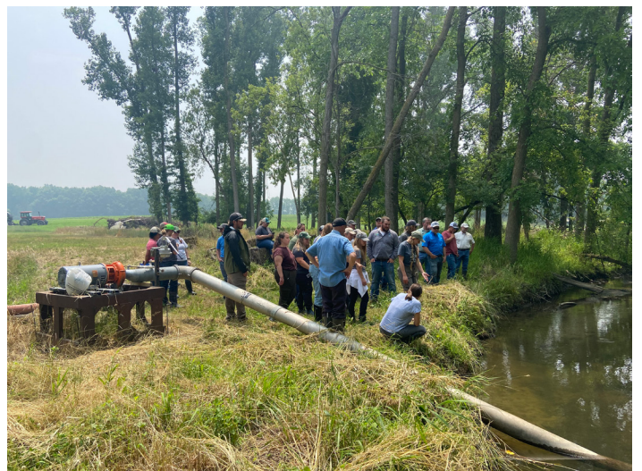
Figure 3. Installed centrifugal pump system pumping from surface water. Michigan State University.
