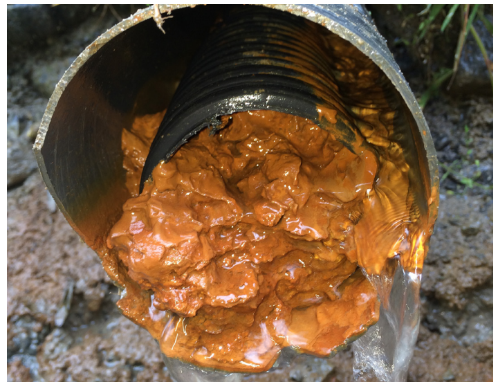
Figure 1- An extreme case of iron ochre deposits inside of a drain pipe (photo credit: Patrick Ruohy)
