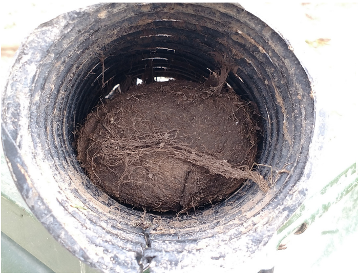
Figure 2- Roots formed a thick bundle that clogged a perforated drain pipe (photo credit: Paul F. Gross).
