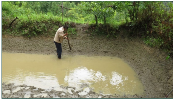
Figure 3-4. Using a pole tied to a gunny bag, a farmer rams and compresses the side wall of a pond.
